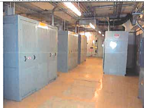
New Electrical Switchgear
